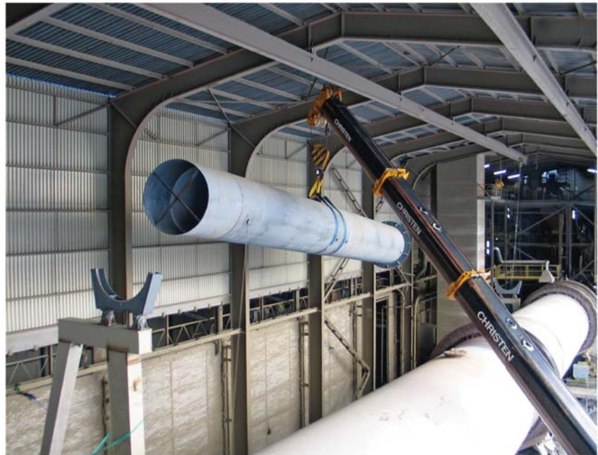
7 Installation of the tertiary air duct during Phase 2 Montage der Tertiärluftleitung in Phase 2
